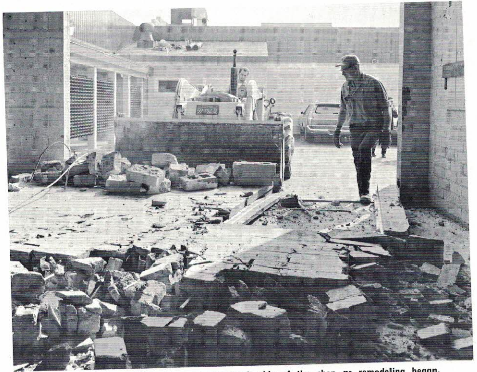
The wall came tumbling down on the south side of the shop as remodeling began.
